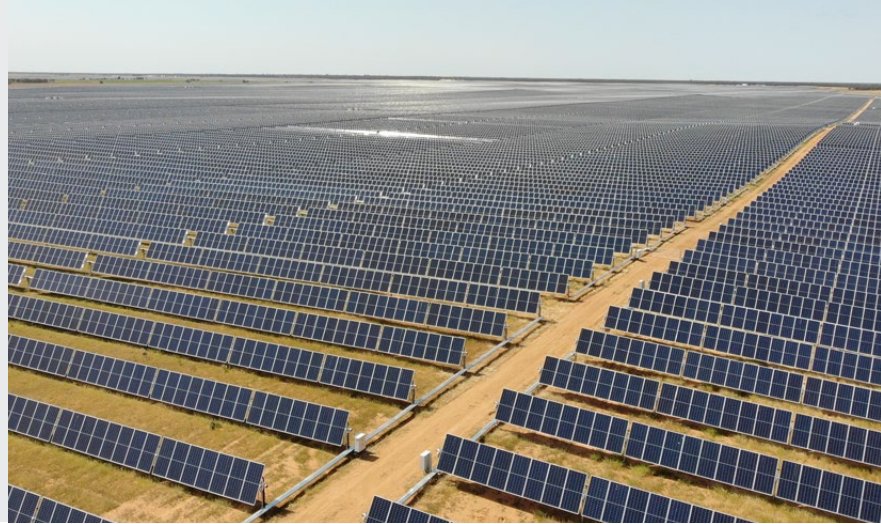
/ Sunraysia Solar Farm, Australia.
